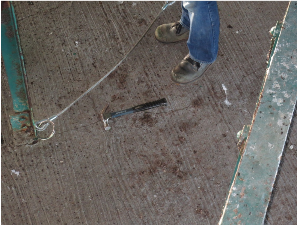
Photo 13: Transverse cracks between truss bearings.
