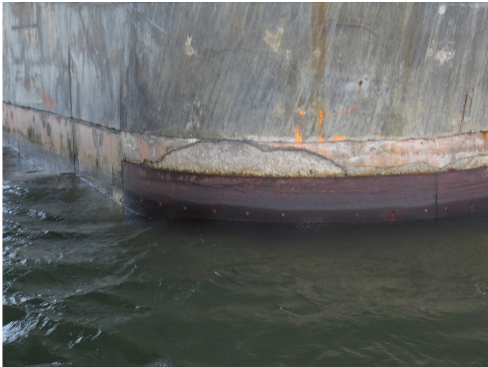
Photo 12: Typical spalling above ice shields.
