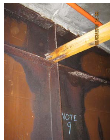
Photo 3.10: Medium Corrosion and Staining Near Cracks in Deck
