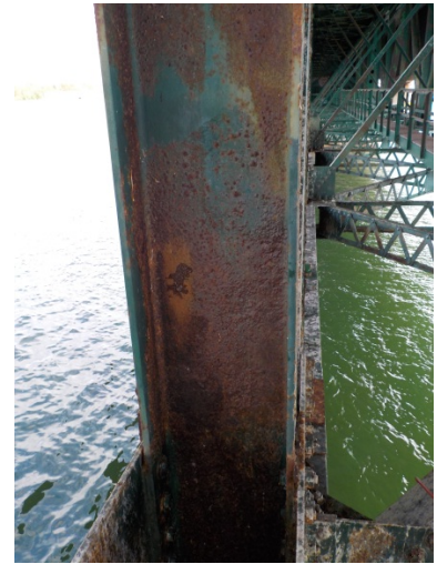
Photo 3.5: Corrosion of Webs and Flanges of Vertical at U16-L16 Left
