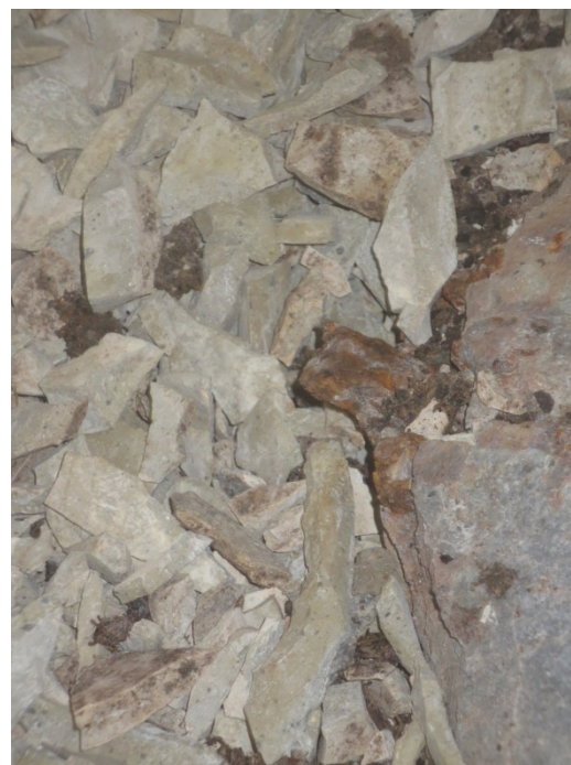
Photo 15: Exposed PT strand.
