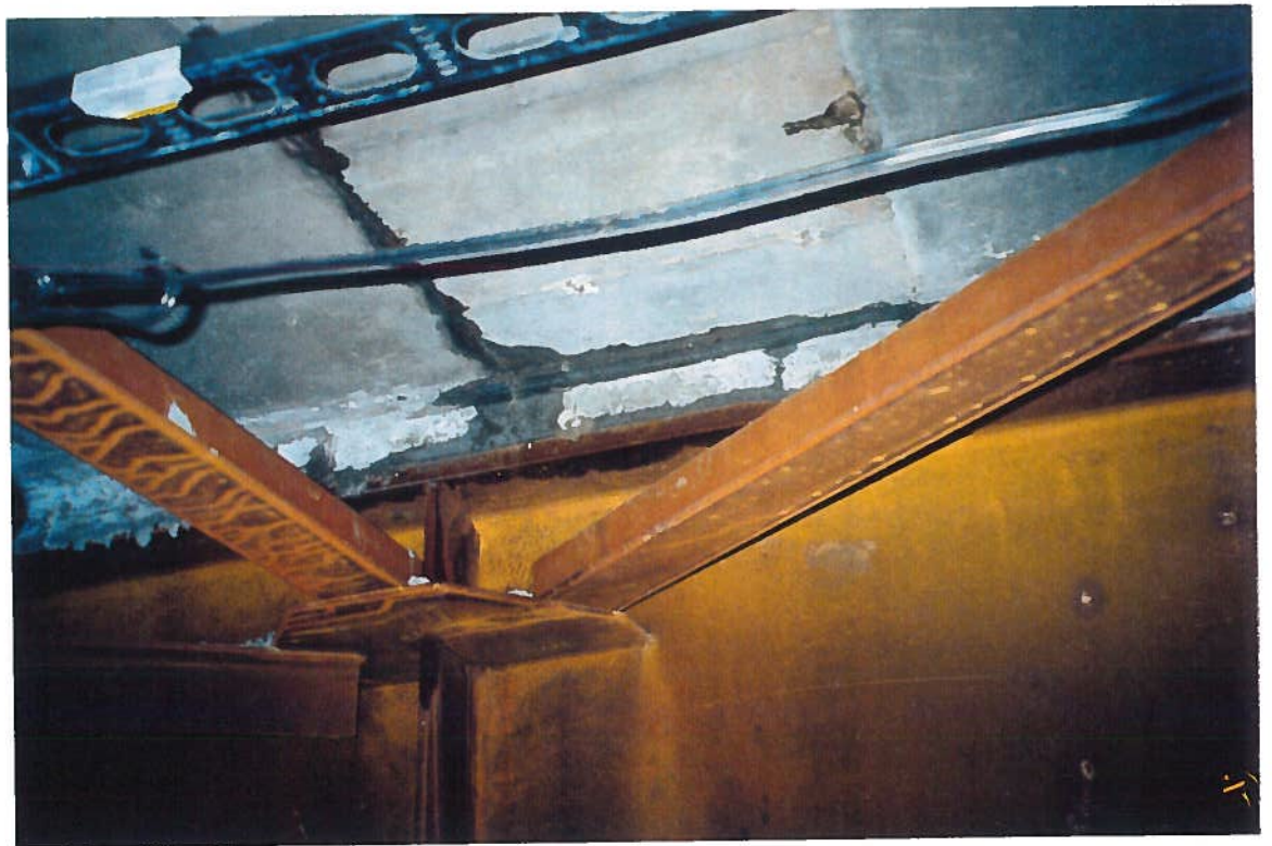
Cracks in precast panels at joints
