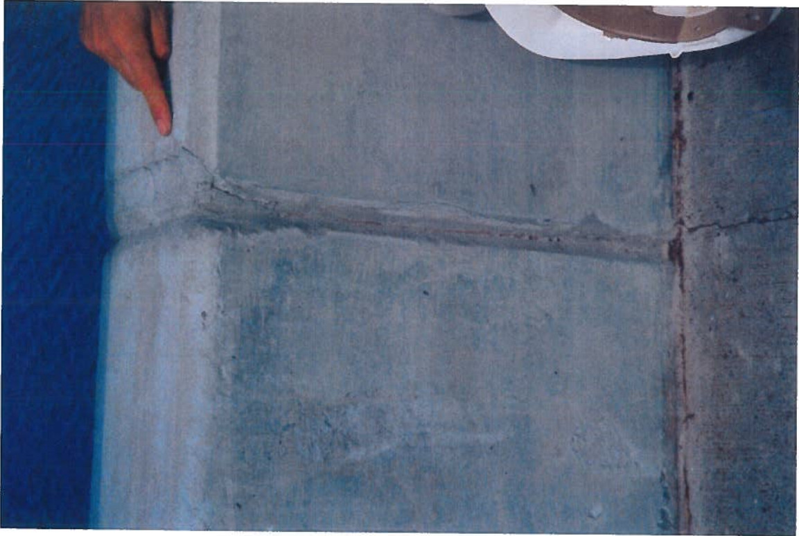
Cracks in parapet close to joints.
