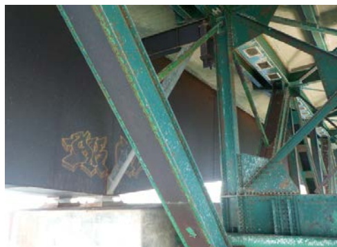
Photo 3.7: Typical Flaking of Coating on Cover Plates
