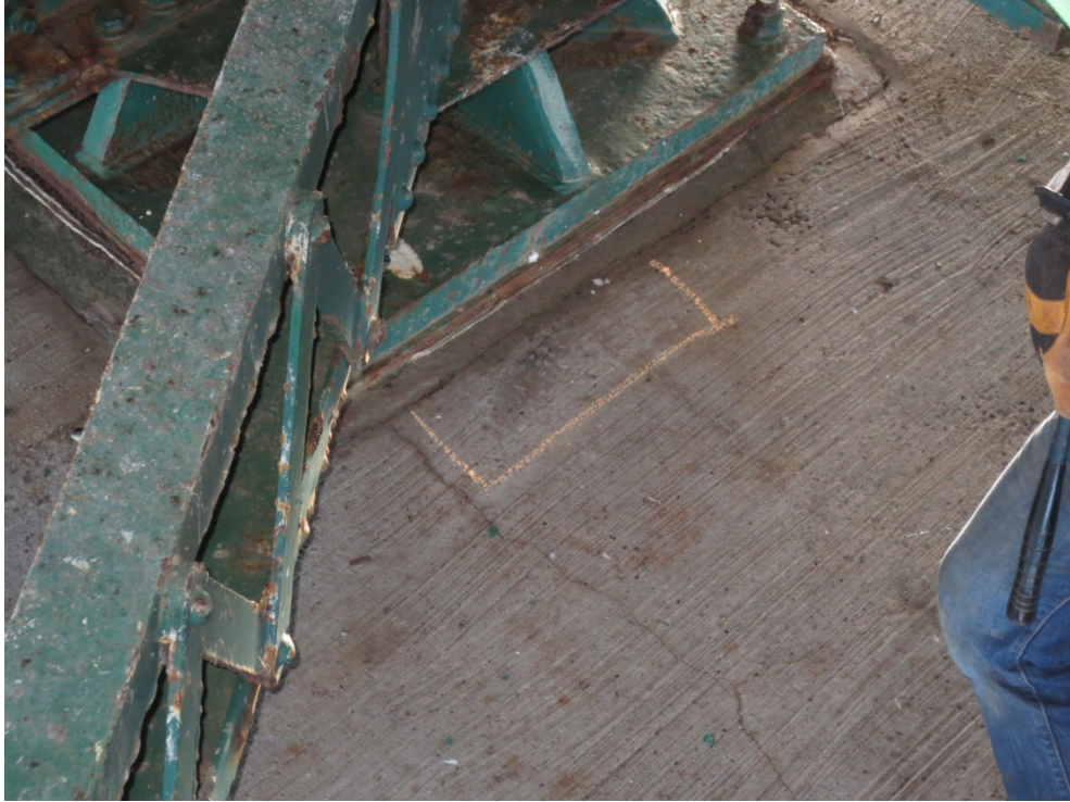
Photo 16: Delamination adjacent to truss bearing.
