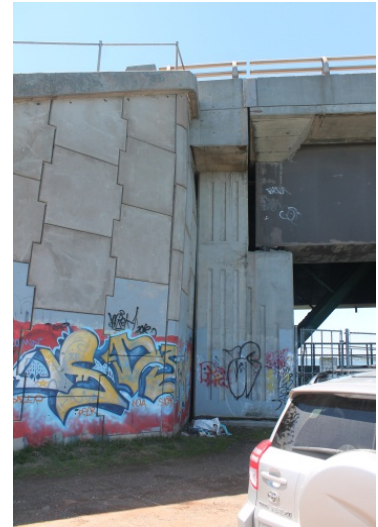
Photo 3.11: Apparent Bulge of MSE Wall at Stratford Abutment
