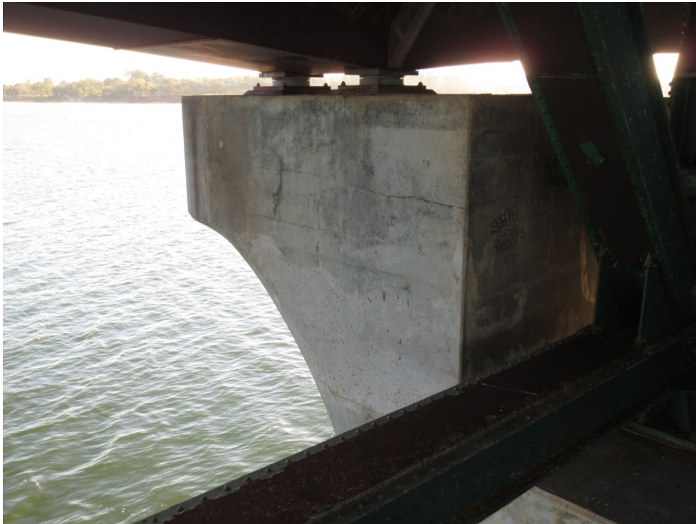
Photo 17: Narrow cracks below box girders.
