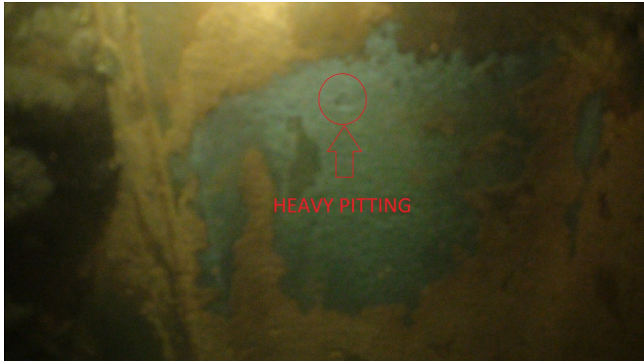
Photo 4: Heavy pitting on SSP.
