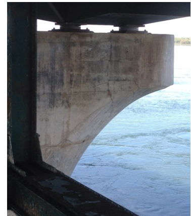
Photo 3.12: Medium Vertical Cracks at Flared Corbel, Typical
