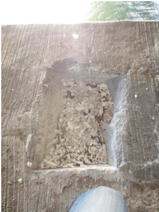
Photo 14: Spalling of grout in post-tensioning block-out.
