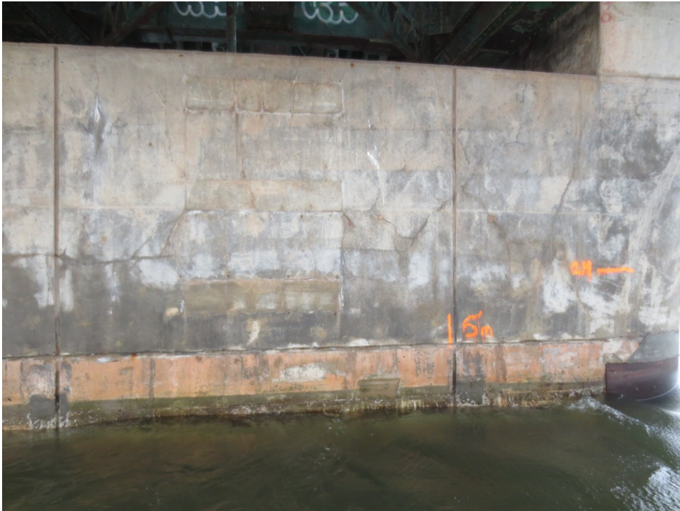
Photo 10: Typical cracking on pier wall.
