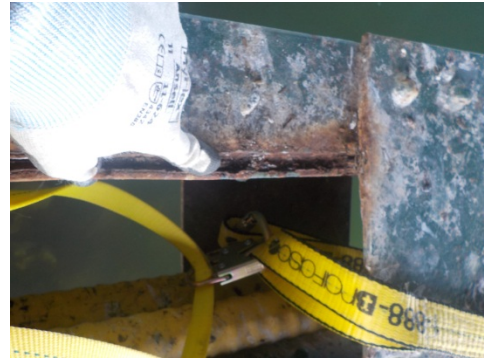
Photo 3.1: Typical Corrosion at Channel/Web Plate Edge
