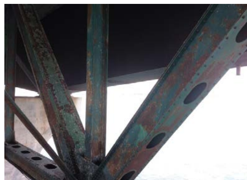
Photo 3.8: Corrosion on Diagonal U13-L14 Left
