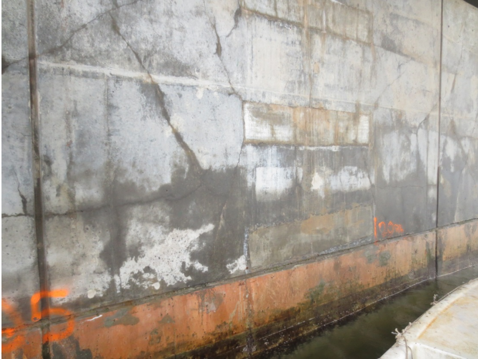
Photo 9: Typical narrow cracking on pier wall.
