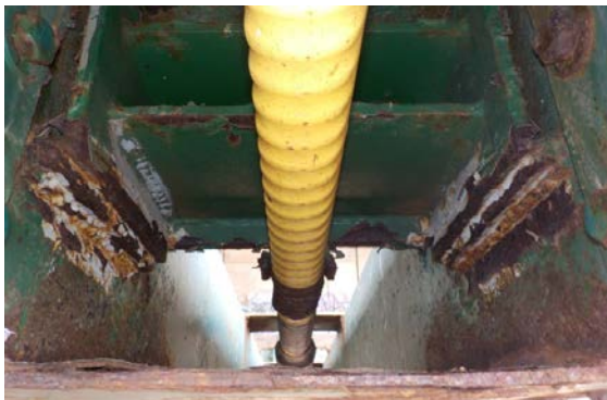
Photo 3.3: Corroded Anchorage of Post Tensioned Reinforcing at L37 Right.
