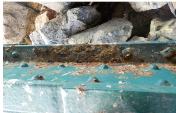
Photo 3.4: Corrosion of the Exterior Bottom Flange at Bottom Chord from L2-L3 Left
