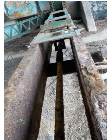
Photo 3.2: Severe Corrosion of Bottom Chords from L39-L37 Right
