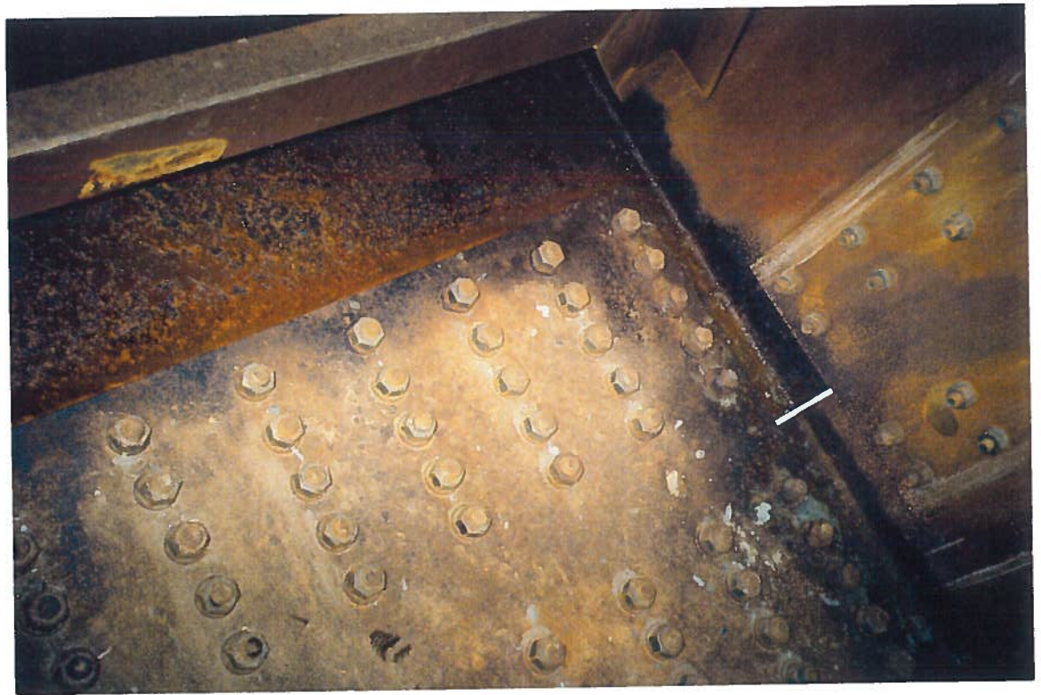
Water at curb face and interior of box
