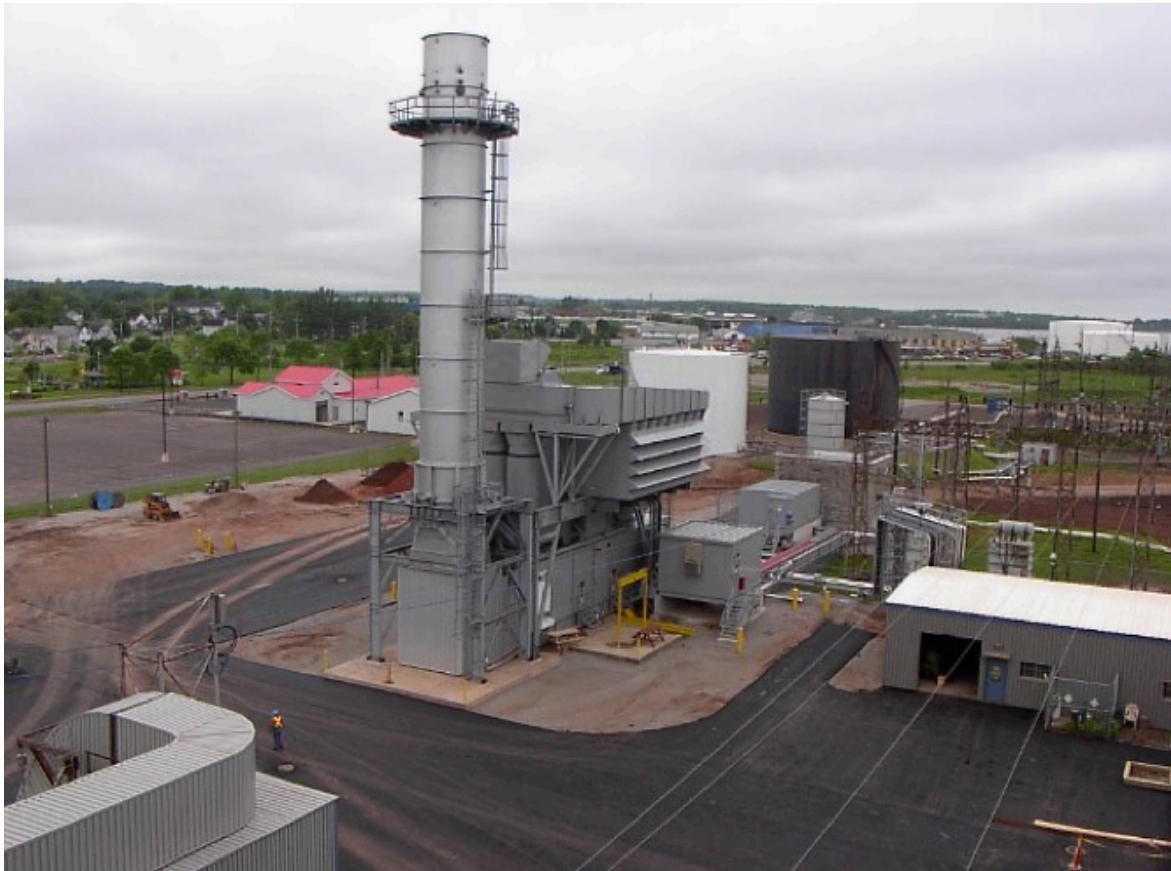
Figure 2.2: Combustion Turbine (CT3) at Maritime Electric's Charlottetown Plant
